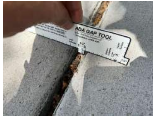
Trip Hazard at Sidewalk Near Building 16 (Critical Repair)
