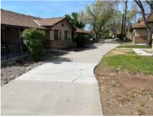
Cracked Sidewalk Near Building 4 (Critical Repair)
