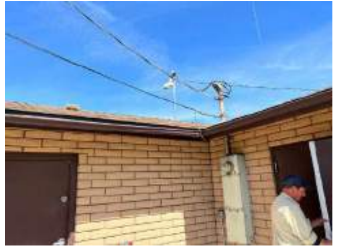
90. Overhead Power Line
