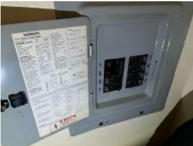
87. Circuit Breaker Panel
