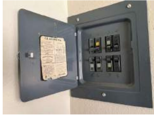
Circuit Breaker Panel (Older)
