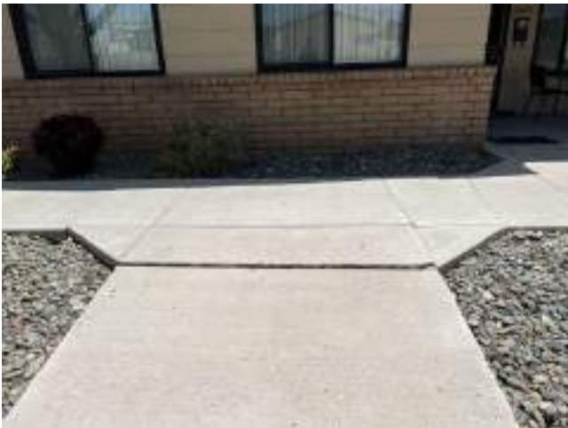
19. Trip Hazard at Sidewalk Near Building 1 (Critical Repair)
