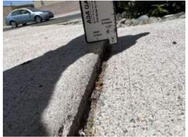
22. Trip Hazard at Sidewalk Near Building 1 (Critical Repair)
