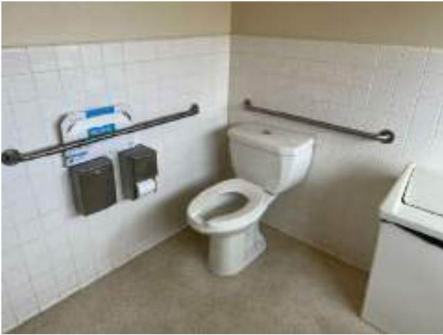
137. Accessible Restroom Toilet
