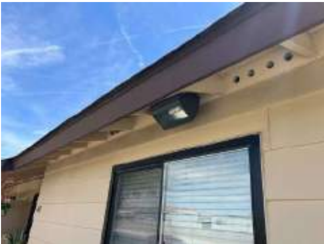
23. Building Mounted Lighting
