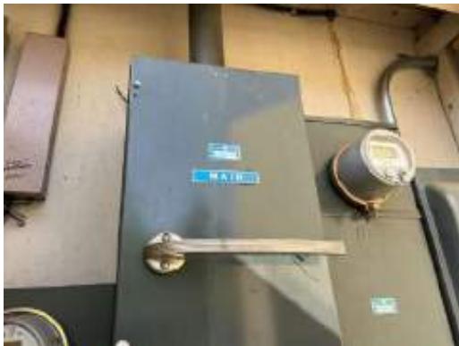
Main Switch Gear
