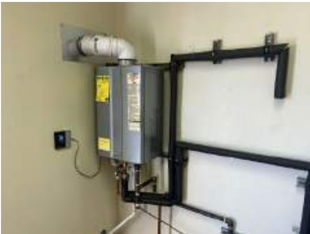
71. Common Area Tankless Water Heater
