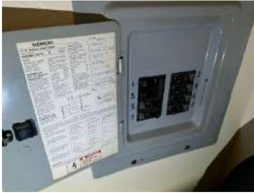
Circuit Breaker Panel
