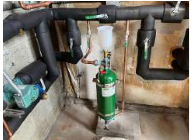
76. Chemical By-Pass Feeder
