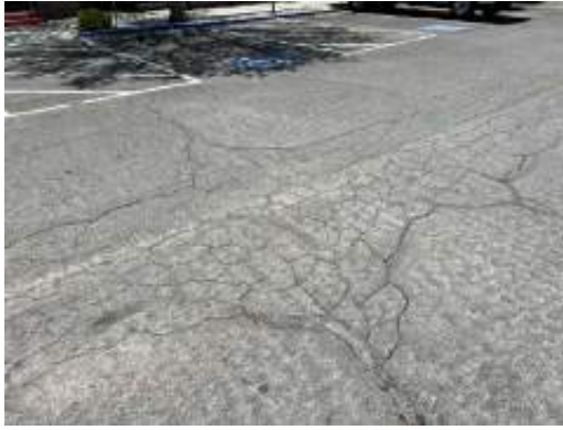
Asphalt Cracking at Community Center Parking Lot (Non-Critical Repair)
