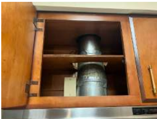
Ducted Hood Vent
