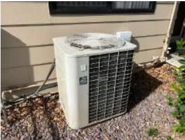
83. Common Area Condensing Unit
