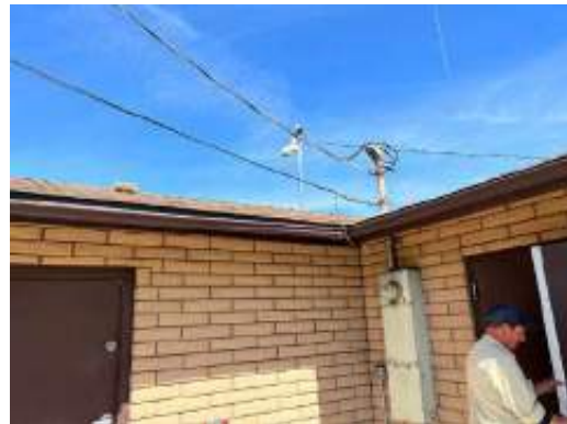
Overhead Power Line
