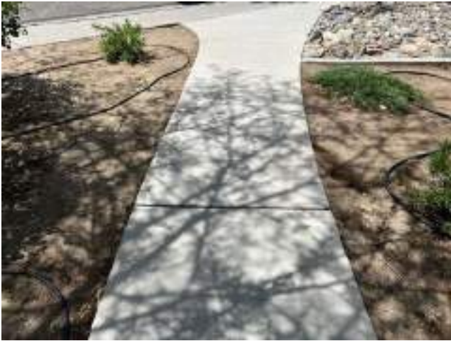
17. Trip Hazard at Sidewalk Near Building 16 (Critical Repair)
