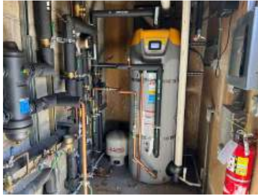
Typical Building Water Heater
