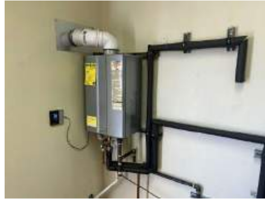
Common Area Tankless Water Heater
