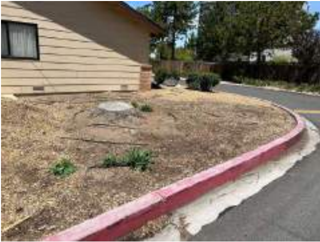
33. Barren Landscaping Near Building 7 (Non-Critical Repair)
