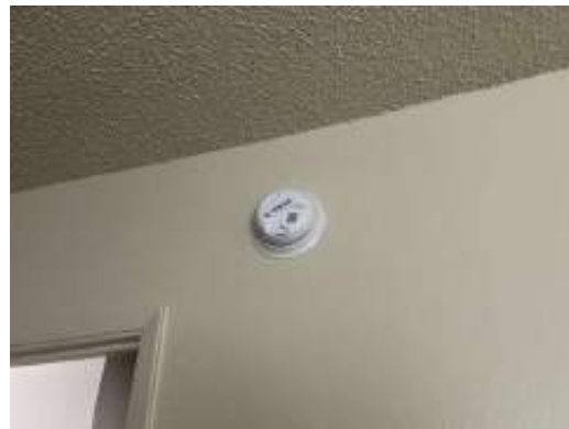
Battery Operated Smoke Detector
