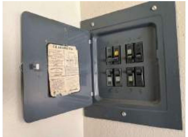
88. Circuit Breaker Panel (Older)
