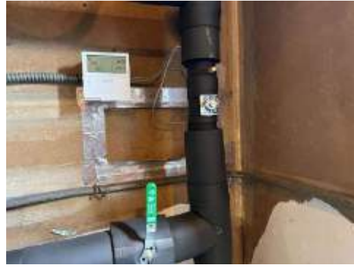
HVAC System Control
