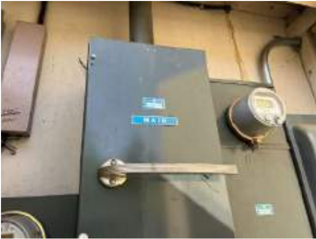
85. Main Switch Gear
