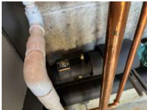
PVC and Copper Piping
