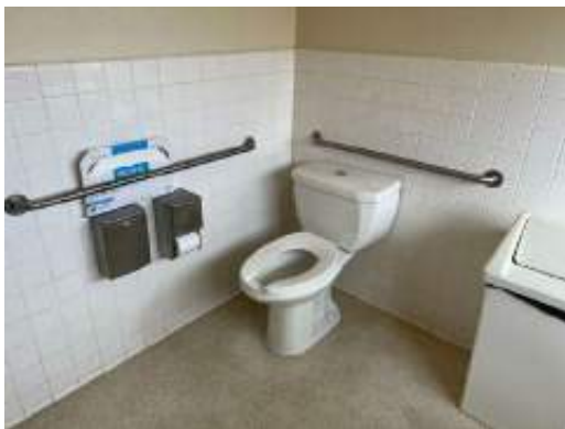
Accessible Restroom Toilet
