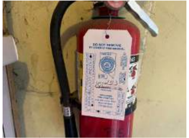
94. Expired Extinguisher Inspection Tag
