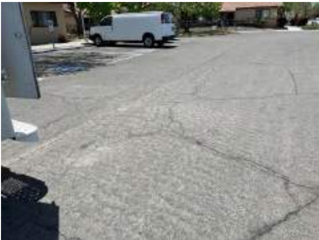
11. Asphalt Cracking at Community Center Parking Lot (Non-Critical Repair)
