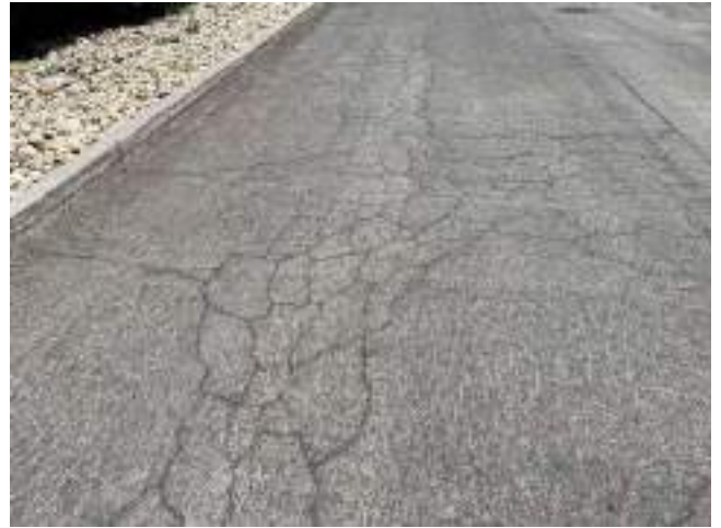
10. Asphalt Condition (Non-Critical Repair)
