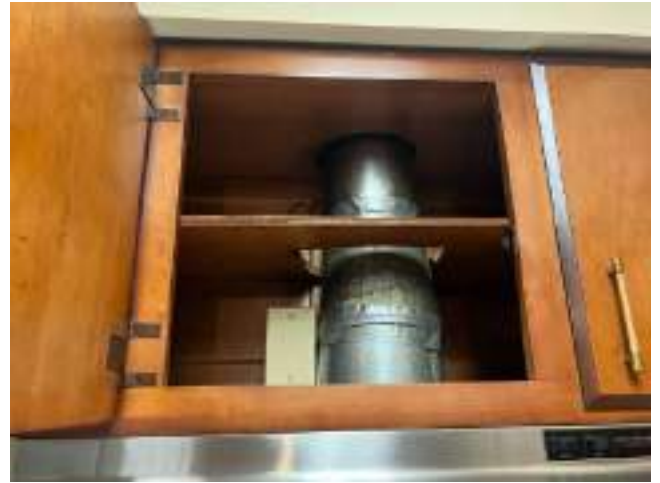
122. Ducted Hood Vent
