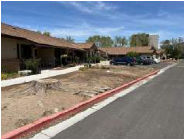
31. Barren Landscaping Near Building 8 (Non-Critical Repair)
