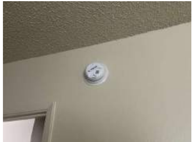
92. Battery Operated Smoke Detector
