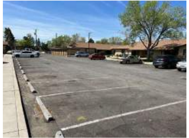
6. Parking Lot - Worn seal coat and faded striping (Non-Critical Repair)
