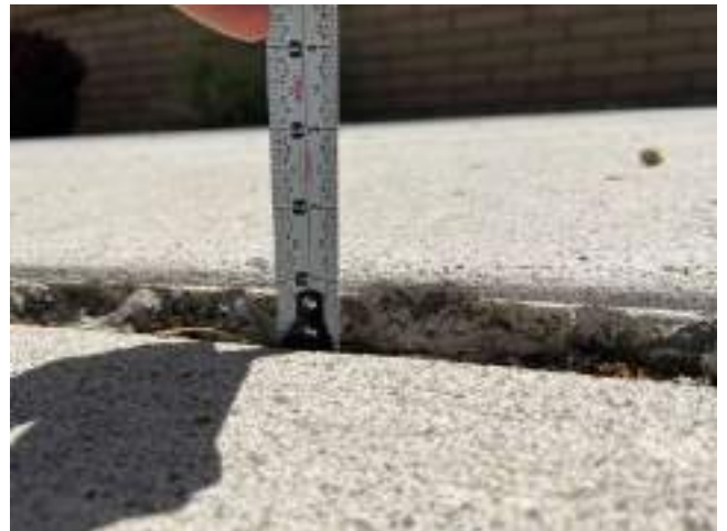
20. Trip Hazard at Sidewalk Near Building 1 (Critical Repair)
