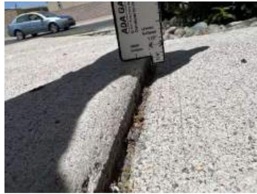
Trip Hazard at Sidewalk Near Building 1 (Critical Repair)
