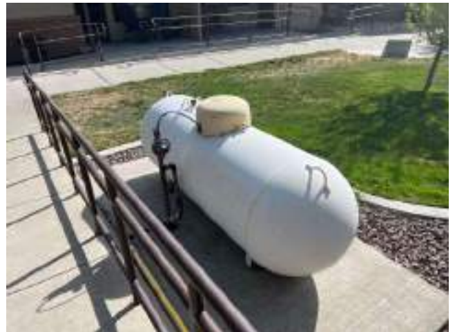
44. Propane Tank for Generator
