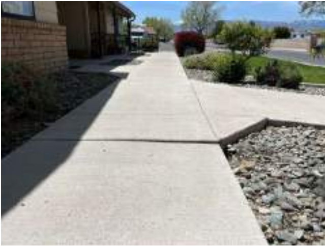
21. Trip Hazard at Sidewalk Near Building 1 (Critical Repair)
