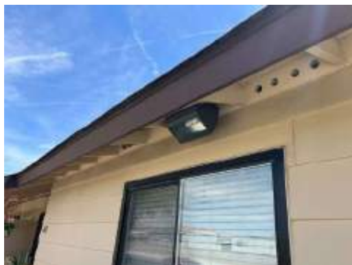
Building Mounted Lighting
