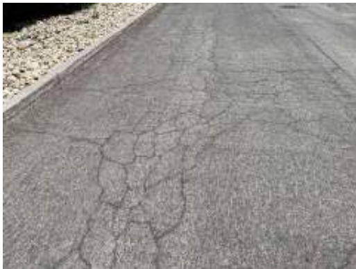
Asphalt Condition (Non-Critical Repair)
