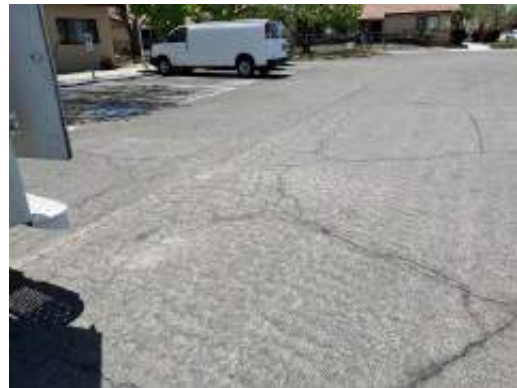
Asphalt Cracking at Community Center Parking Lot (Non-Critical Repair)
