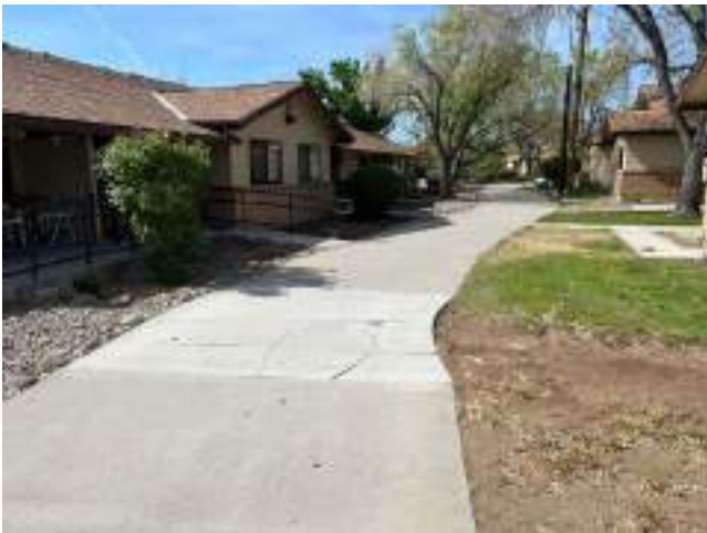
15. Cracked Sidewalk Near Building 4 (Critical Repair)
