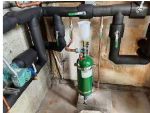
Chemical By-Pass Feeder
