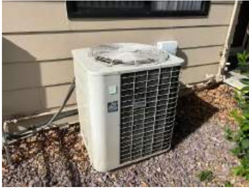
Common Area Condensing Unit
