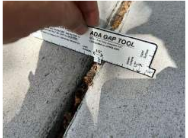
18. Trip Hazard at Sidewalk Near Building 16 (Critical Repair)
