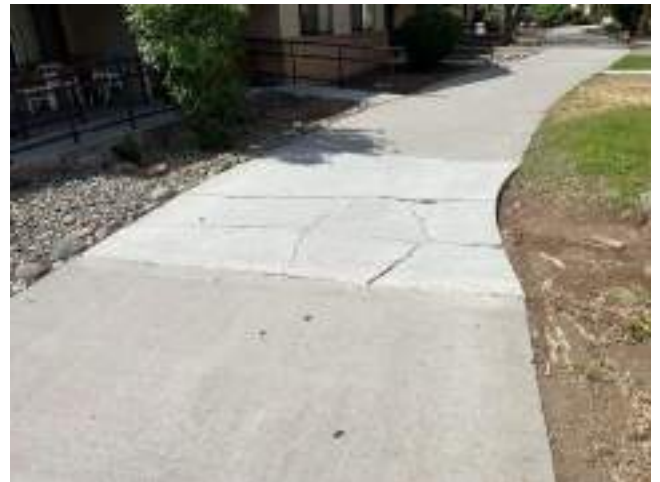
16. Cracked Sidewalk Near Building 4 (Critical Repair)
