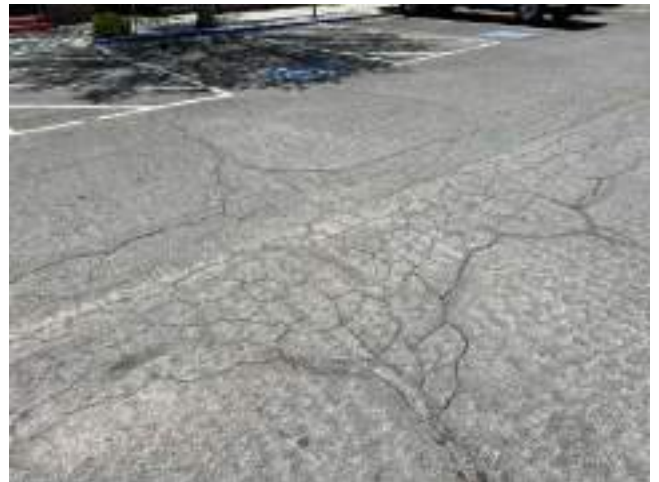
12. Asphalt Cracking at Community Center Parking Lot (Non-Critical Repair)
