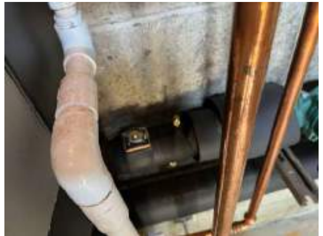
72. PVC and Copper Piping
