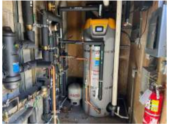
70. Typical Building Water Heater
