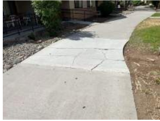
Cracked Sidewalk Near Building 4 (Critical Repair)
