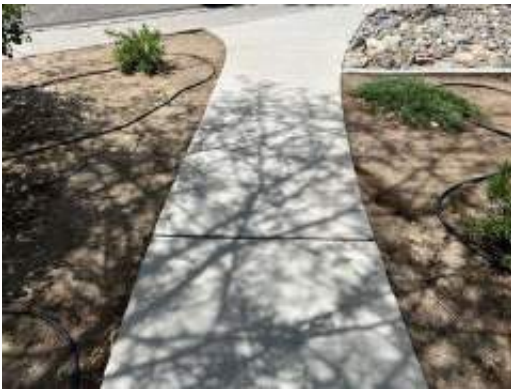
Trip Hazard at Sidewalk Near Building 16 (Critical Repair)
