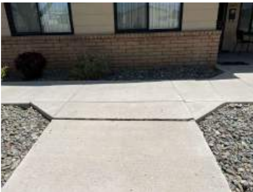
Trip Hazard at Sidewalk Near Building 1 (Critical Repair)
