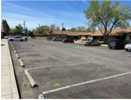
Parking Lot - Worn seal coat and faded striping (Non-Critical Repair)
