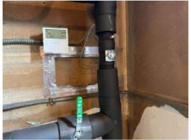
78. HVAC System Control
