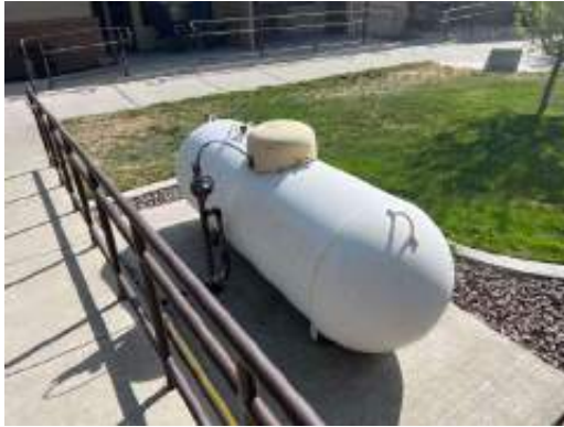
Propane Tank for Generator
