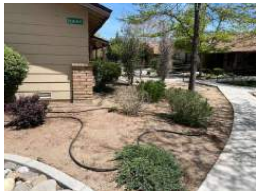
Barren Landscaping Near Building 16 (Non-Critical Repair)
