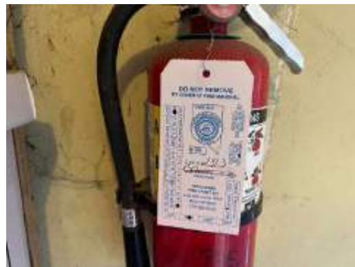
Expired Extinguisher Inspection Tag
