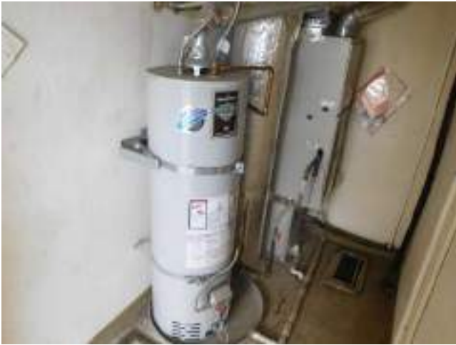
161. Typical nat gas fired water heater and furnace
