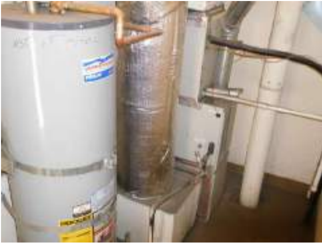
165. Typical nat gas fired water heater and furnace
