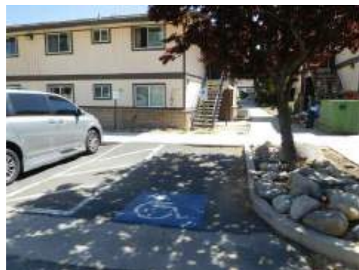
Typical ADA parking space at UFAS dwelling unit excessive slope and cross slope at access ramp (Critical Repair)
