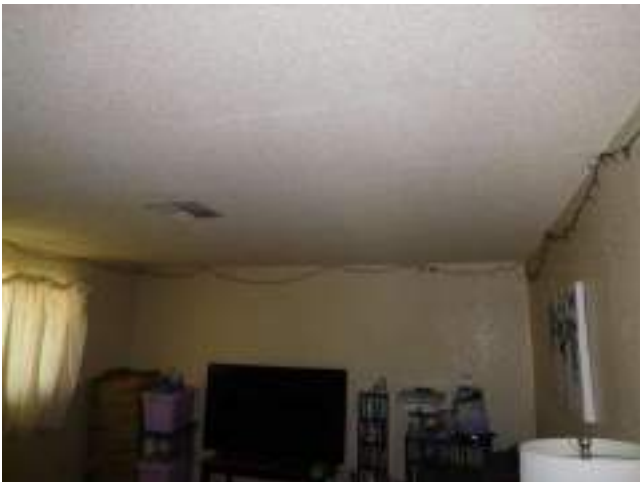
143. Typical drywall damage from building settling
