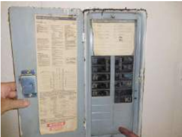
15. Bld 1512-Unit 3-2x1 -Breaker panel
