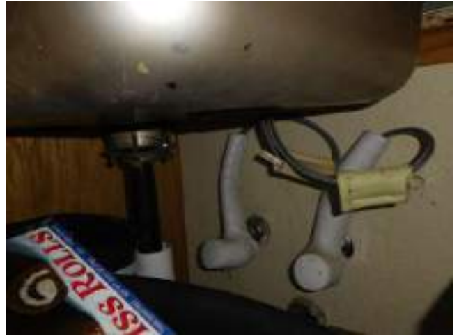
54. Bld 2541-Unit 1-2x1-UFAS -Kitchen partial scald and abrasion protection (Critical Repair)
