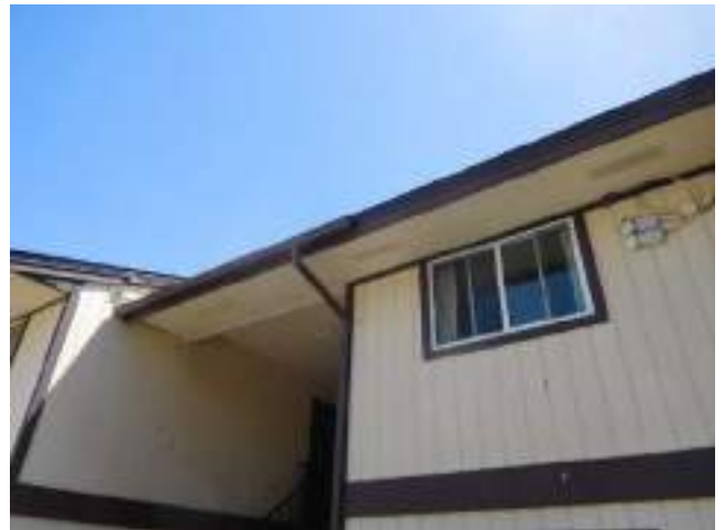
160. Conjoined covered entry gutter and downspout
