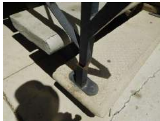
Upper floor unit access stairway at 1516 building damaged hand railing (Critical Repair)
