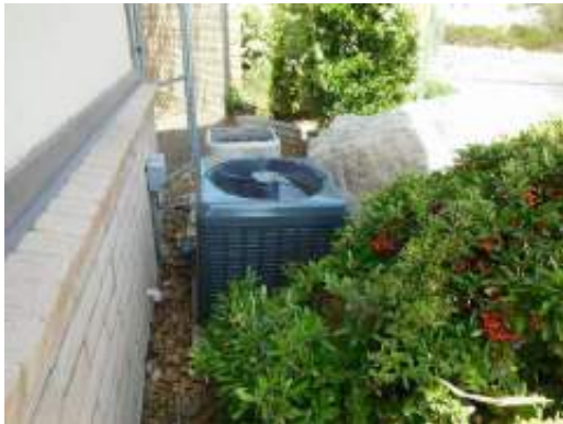
Exterior condensing unit
