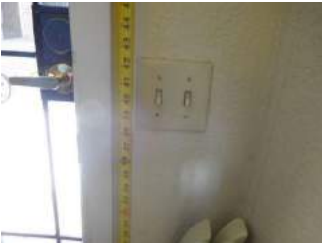
19. Bld 2541-Unit 1-2x1-UFAS -Typical wall switch height
