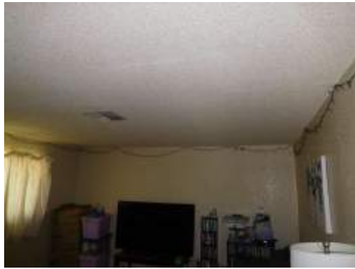
Typical drywall damage from building settling
