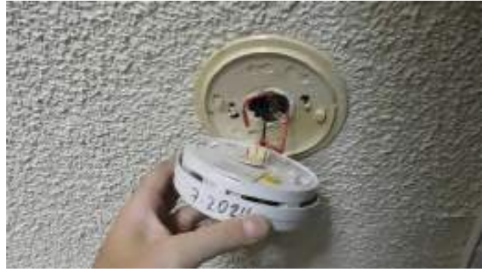
178. Typical dwelling unit hardwired smoke detection
