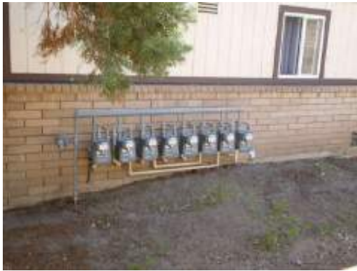
Typical dwelling unit Nat Gas metering
