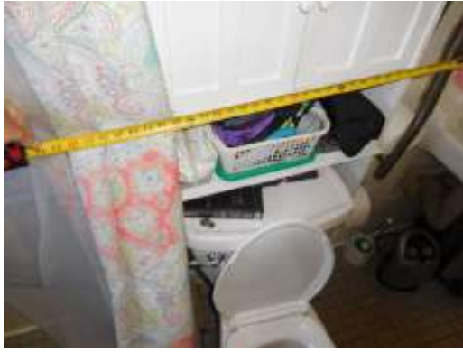
Bld 2541-Unit 1-2x1-UFAS -Bathroom inadequate clear space at toilet (Critical Repair)
