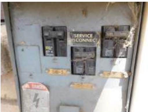
Typical dwelling unit metered service 100-amp main breaker
