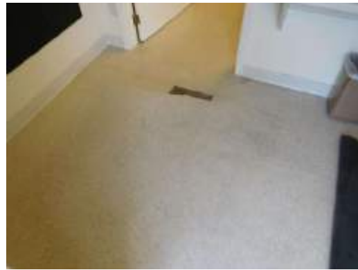
Leasing Office entrance slab uplift and movement
