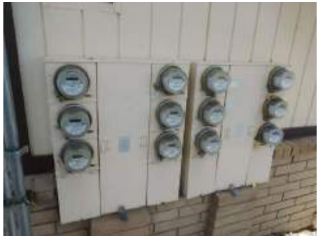
96. Typical dwelling unit electric metering
