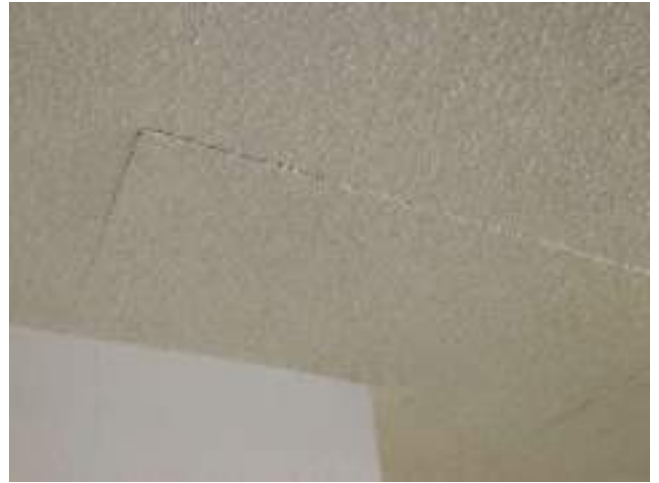
54. Leasing Office Community Room evidence of movement
