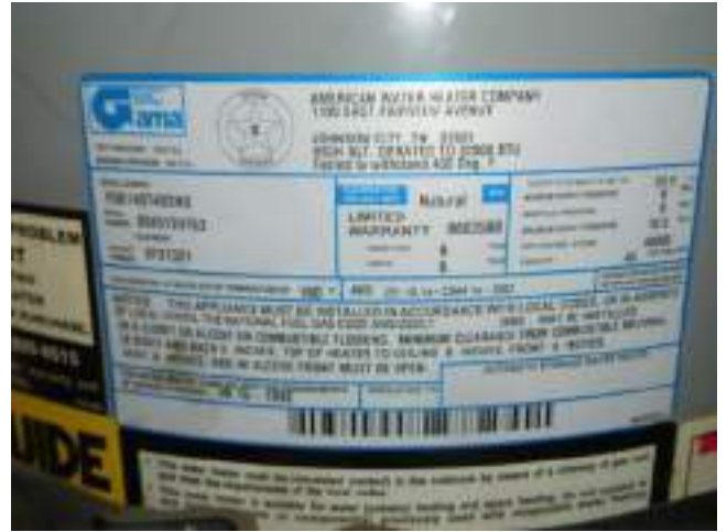
166. Water heater tagging
