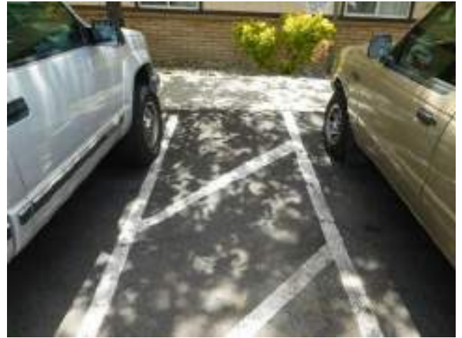
74. Typical ADA parking space at UFAS dwelling unit excessive slope and cross slope at access ramp (Critical Repair)
