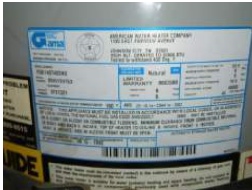
Water heater tagging
