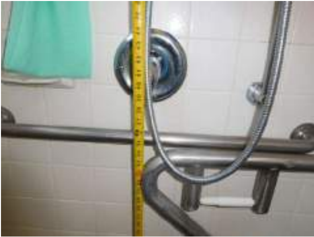
30. Bld 2541-Unit 1-2x1-UFAS -Bathroom
