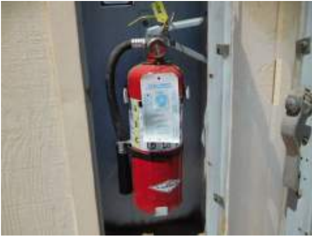
181. Typical fire extinguisher
