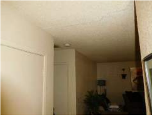
141. Typical drywall damage from building settling
