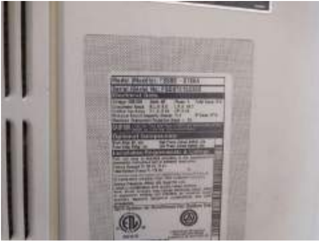
173. Exterior condensing unit tagging
