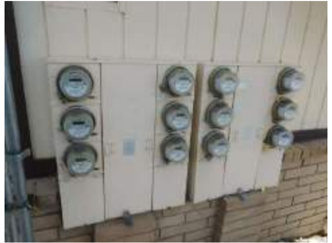
174. Typical dwelling unit meter bank
