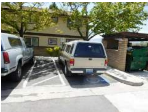
Typical ADA parking space at UFAS dwelling unit excessive slope and cross slope at access ramp (Critical Repair)
