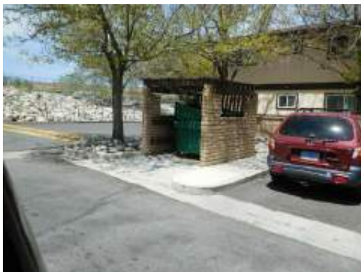
Refuse container with no accessible pathway (Critical Repair)
