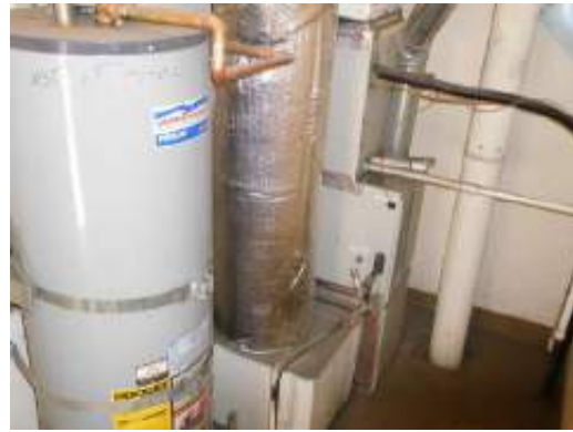
Typical nat gas fired water heater and furnace
