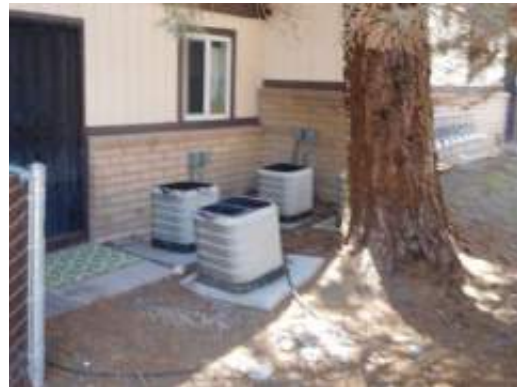
Exterior condensing units
