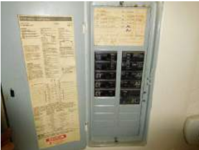
175. Typical dwelling unit ITE breaker panel
