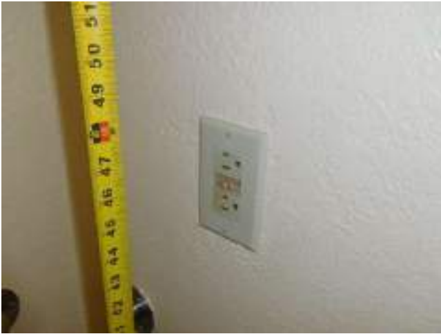
53. Leasing Office Community Room bathroom GFIC
