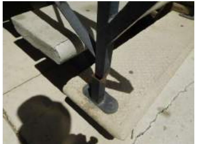
100. Upper floor unit access stairway at 1516 building damaged hand railing (Critical Repair)
