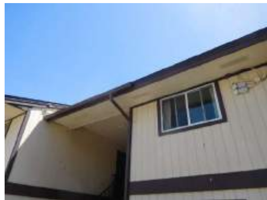
Conjoined covered entry gutter and downspout
