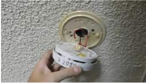
Typical dwelling unit hardwired smoke detection
