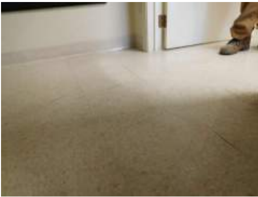
Leasing Office entrance slab uplift and movement
