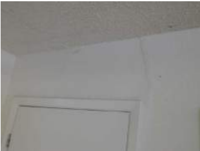
55. Leasing Office Community Room evidence of movement
