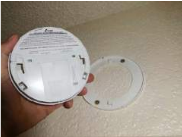
179. Typical dwelling unit battery operated smoke detection
