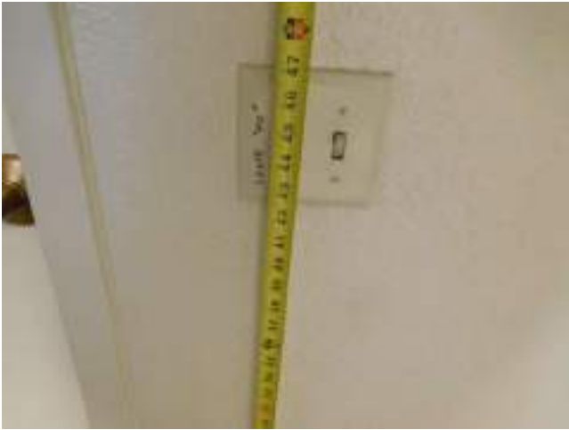
29. Leasing Office Community Room lighting controls
