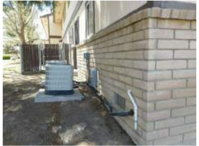
170. Exterior condensing units
