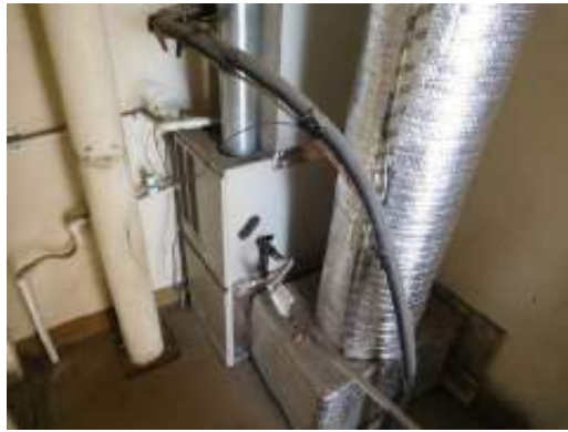
Typical nat gas fired water heater and furnace
