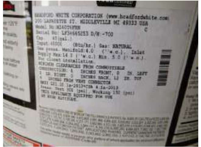
162. Water heater tagging
