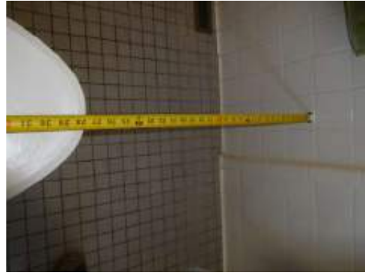
Bld 2541-Unit 1-2x1-UFAS -Bathroom inadequate clear space at toilet (Critical Repair)
