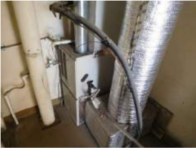
169. Typical nat gas fired water heater and furnace
