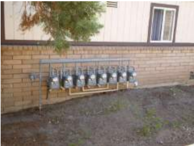
95. Typical dwelling unit Nat Gas metering
