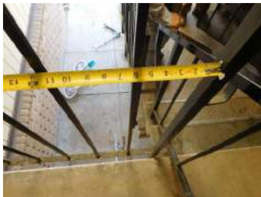
Typical onsite railing system with excessive bollard opening widths (Critical Repair)
