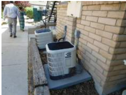
Exterior condensing units
