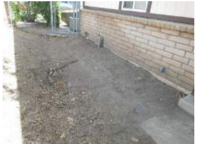
120. Site stormwater drainage
