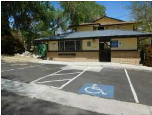
Laundry room with non-compliant access pathway from accessible space (Critical Repair)
