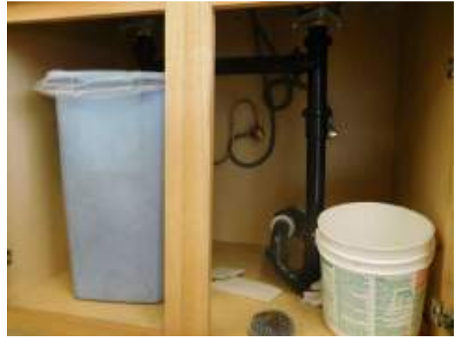
34. Leasing Office Community Room Kitchen non accessible kitchen sink
