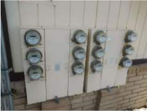
Typical dwelling unit meter bank
