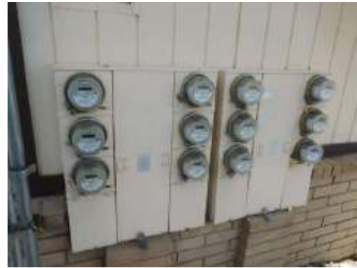
Typical dwelling unit electric metering
