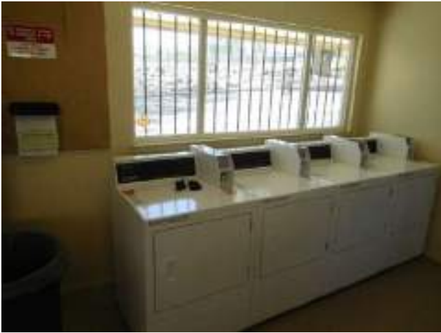
93. Laundry Room dryers
