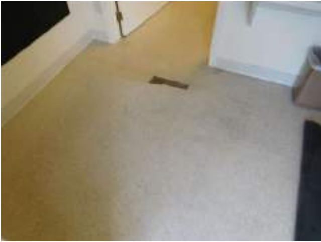
57. Leasing Office entrance slab uplift and movement
