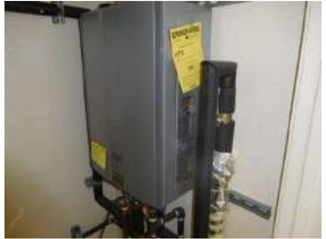
90. Laundry Room tankless water heater
