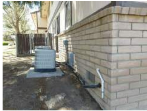
Exterior condensing units
