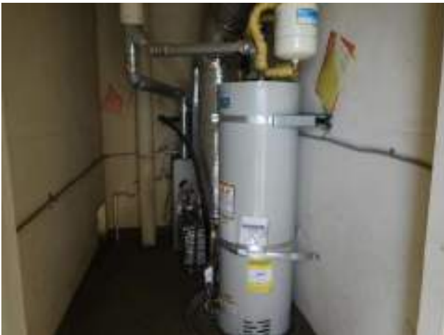
167. Typical nat gas fired water heater and furnace
