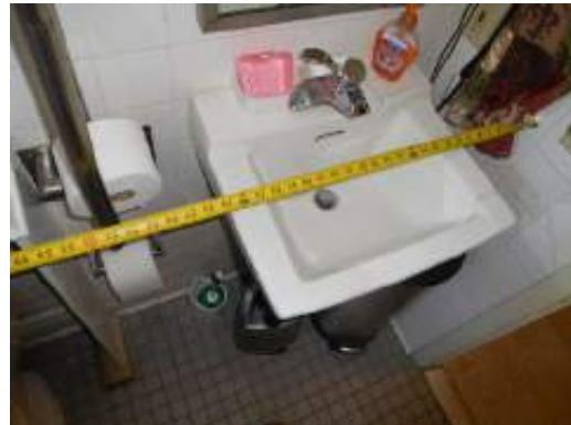
Bld 2541-Unit 1-2x1-UFAS -Bathroom inadequate clear space at sink (Critical Repair)
