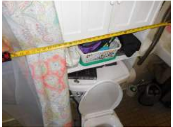
26. Bld 2541-Unit 1-2x1-UFAS -Bathroom inadequate clear space at toilet (Critical Repair)
