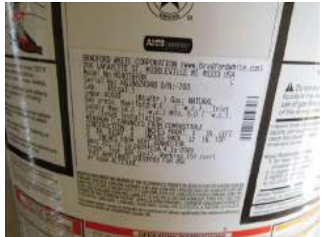
168. Water heater tagging
