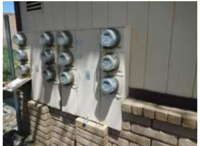
176. Typical dwelling unit meter bank
