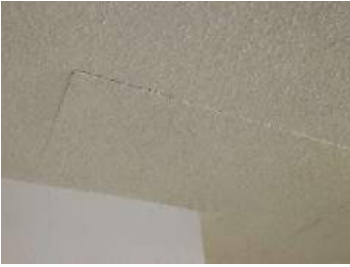
Leasing Office Community Room evidence of movement
