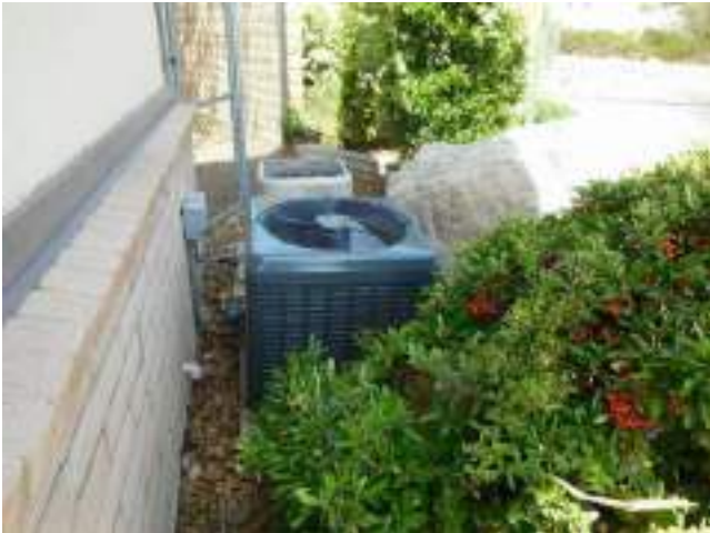
163. Exterior condensing unit
