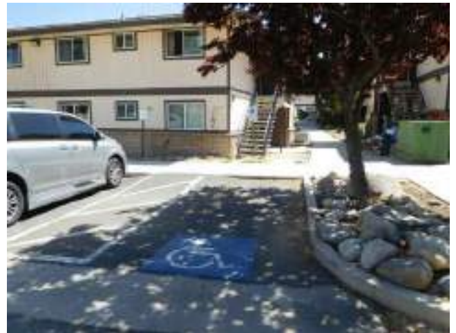
76. Typical ADA parking space at UFAS dwelling unit excessive slope and cross slope at access ramp (Critical Repair)
