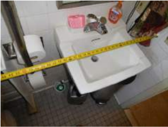
25. Bld 2541-Unit 1-2x1-UFAS -Bathroom inadequate clear space at sink (Critical Repair)
