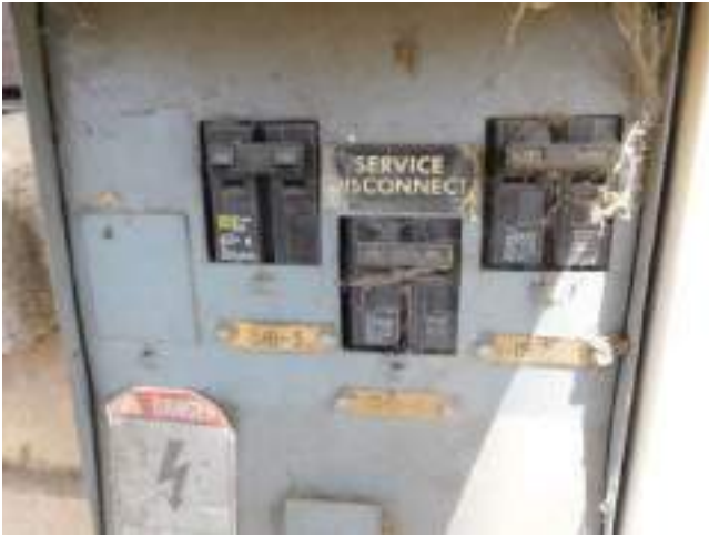
177. Typical dwelling unit metered service 100-amp main breaker
