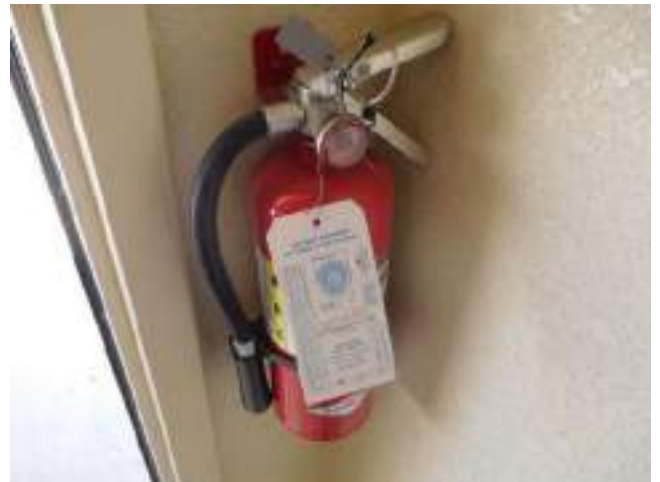
180. Typical fire extinguisher
