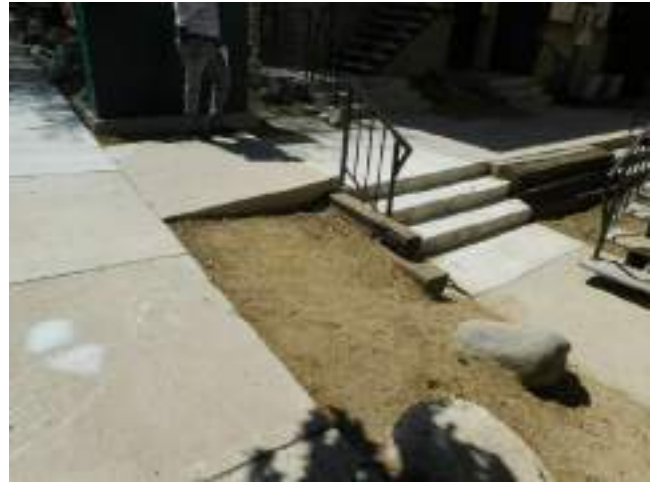
82. Site stairway and sectional uplift trip hazard between 1512 and 1504 Buildings, single hand railing at 3 site stairways (Critical Repair)
