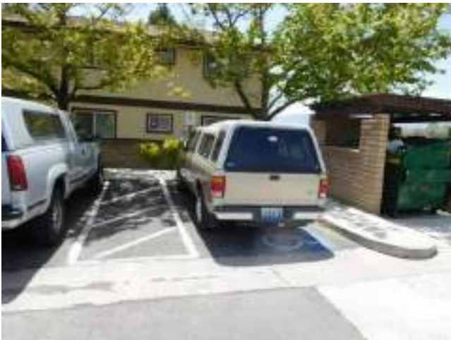
75. Typical ADA parking space at UFAS dwelling unit excessive slope and cross slope at access ramp (Critical Repair)
