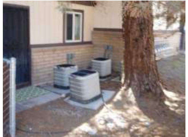
164. Exterior condensing units
