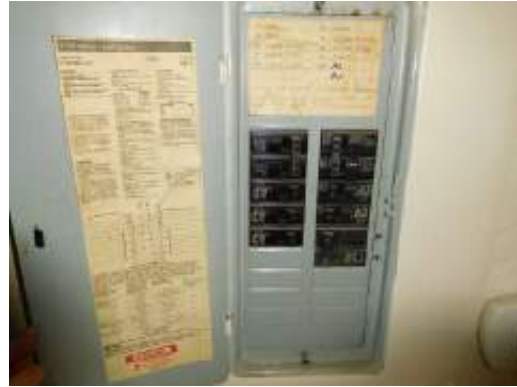
Typical dwelling unit ITE breaker panel
