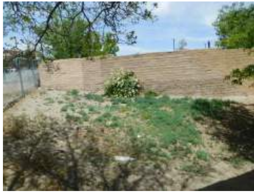
Partially retaining site wall at northern end of site, area of recent sectional replacement
