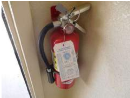
Typical fire extinguisher
