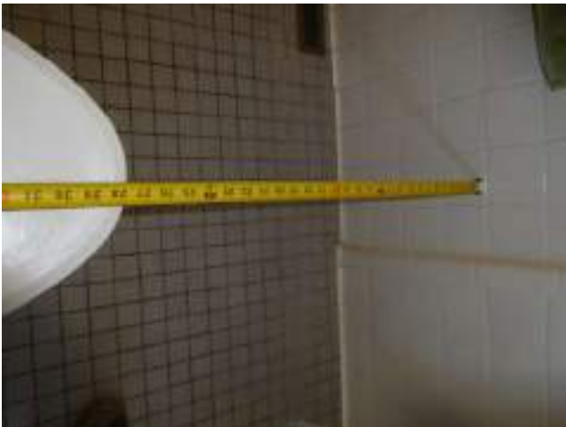
27. Bld 2541-Unit 1-2x1-UFAS -Bathroom inadequate clear space at toilet (Critical Repair)
