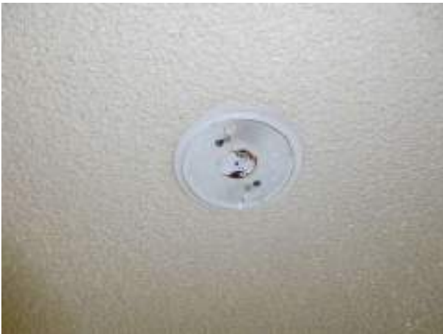
7. Bld 1512-Unit 3-2x1 -Bedroom hardwired smoke detection
