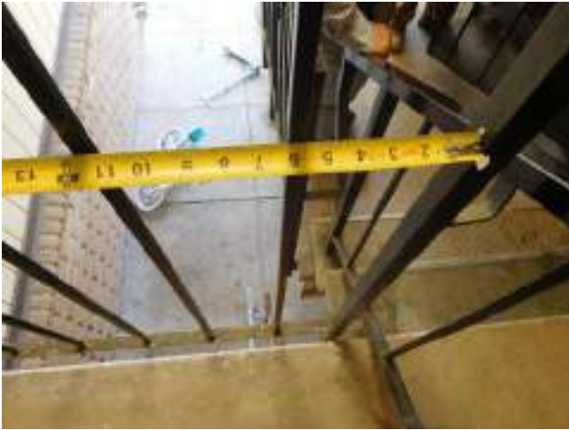
105. Typical onsite railing system with excessive bollard opening widths (Critical Repair)
