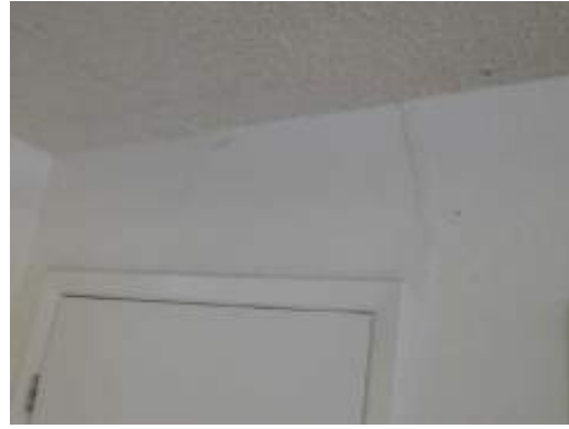
Leasing Office Community Room evidence of movement
