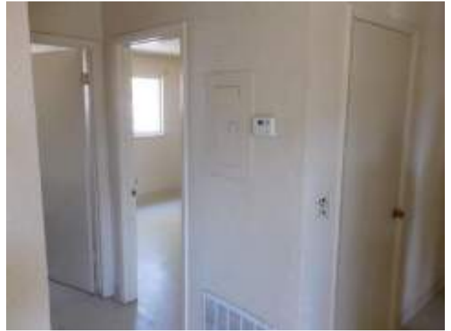
10. Bld 1512-Unit 3-2x1 -Hall with breaker panel and thermostat
