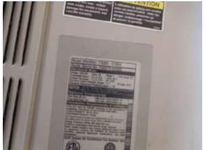
172. Exterior condensing unit tagging
