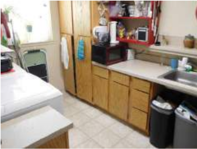
53. Bld 2541-Unit 1-2x1-UFAS -Kitchen missing cabinet and drawer handles/pulls (Critical Repair)
