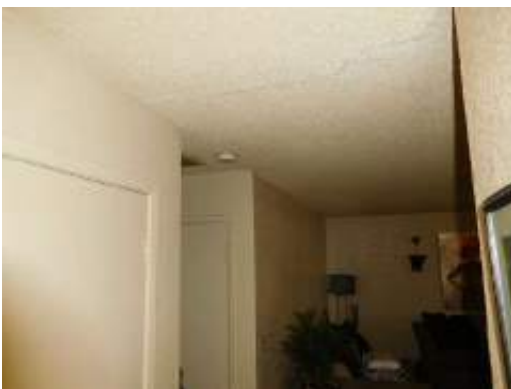
Typical drywall damage from building settling
