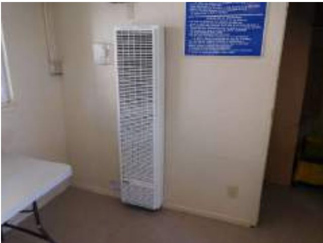
91. Laundry Room nat gas wall heater
