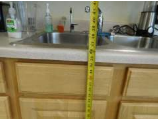
35. Leasing Office Community Room Kitchen non accessible kitchen sink
