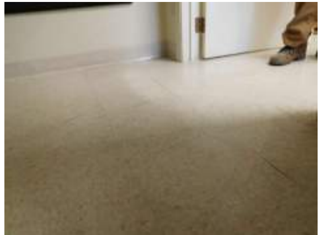
56. Leasing Office entrance slab uplift and movement
