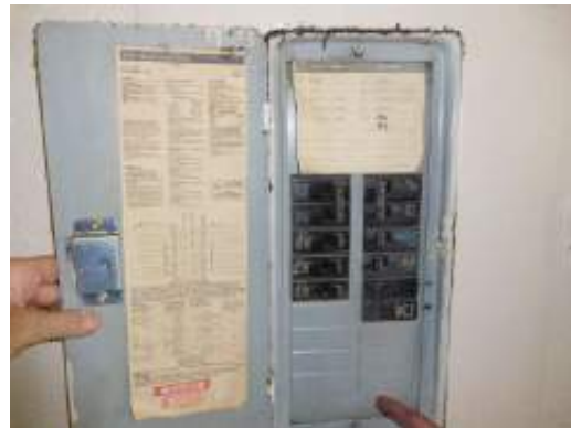
Bld 1512-Unit 3-2x1 -Breaker panel
