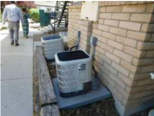
171. Exterior condensing units
