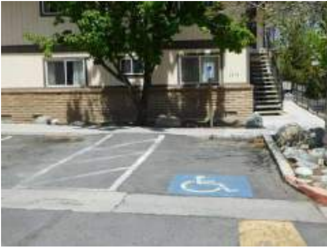
77. Typical ADA parking space at UFAS dwelling unit excessive slope and cross slope at access ramp (Critical Repair)
