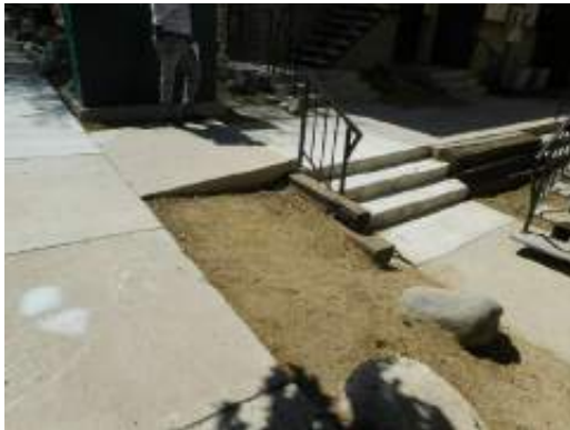
Site stairway and sectional uplift trip hazard between 1512 and 1504 Buildings, single hand railing at 3 site stairways (Critical Repair)
