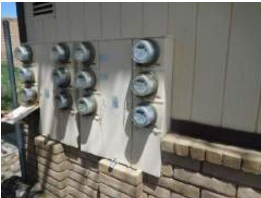
Typical dwelling unit meter bank
