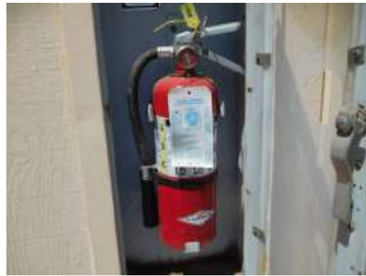
Typical fire extinguisher
