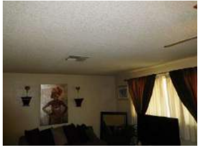
142. Typical drywall damage from building settling
